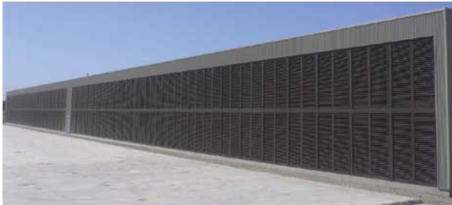
An exterior view of the Advanced Data Centers facility in Sacramento, Calif.
